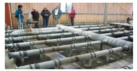
Figure 18: Wastewater is sprayed onto a grill coated with bacteria that absorb dissolved organic matter and trap particles.
