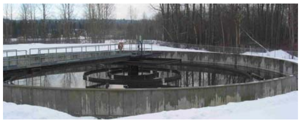
Figure 19. More solids settle out in large tanks (clarifiers).
