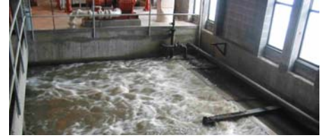
Figure 17. Wastewater arriving at the treatment plant. Solids are trapped and removed on screens.
